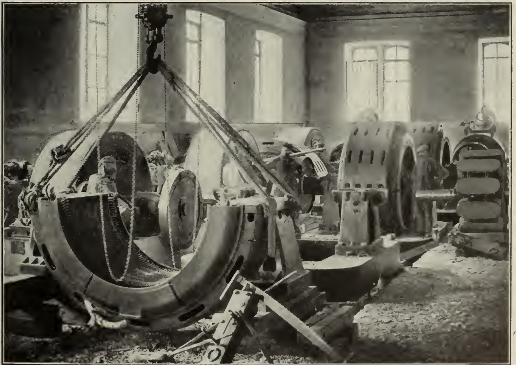
PARTLY ERECTED ALTERNATORS IN THE NOVALESA STATION.
